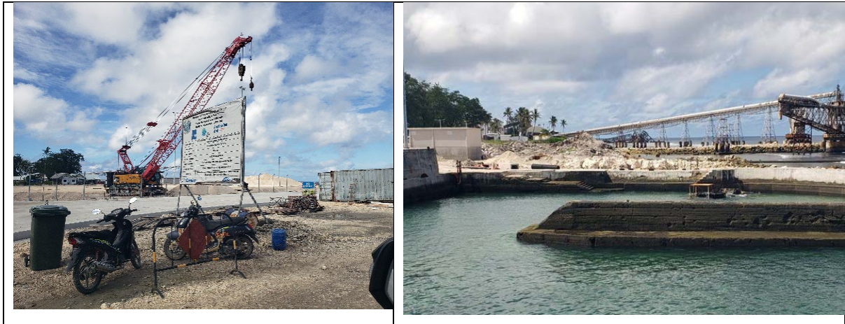
Figure 17-11 Construction works at the port (left) Cantilever conveyor used for loading phosphate onto carrier ships (right). Photo credit: CSIRO, 2024.
