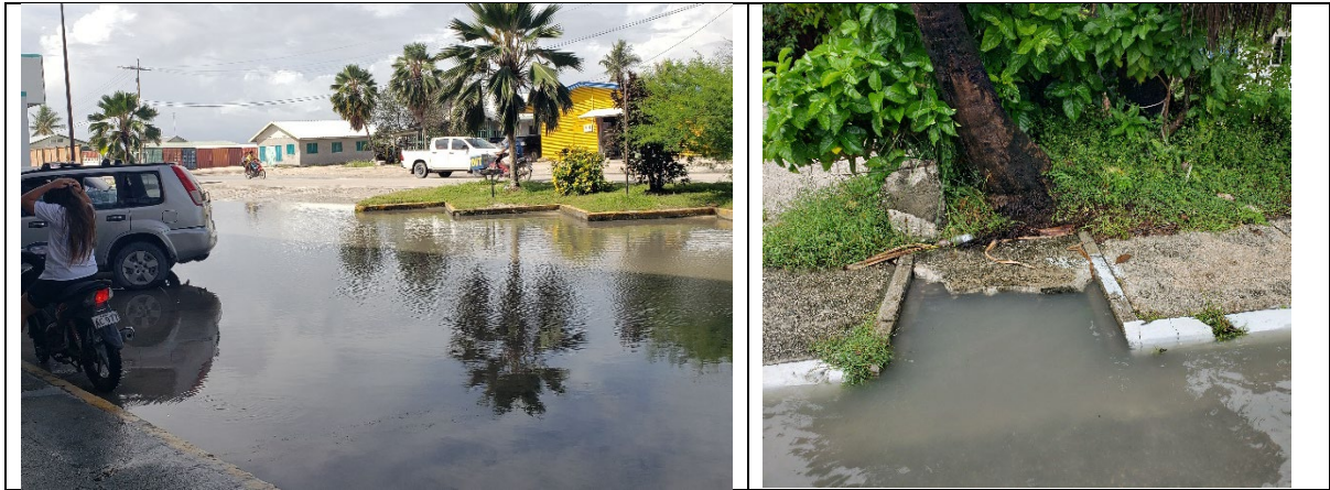
Figure 17-5 Flooded carpark after heavy rain (left) and blocked drain (right). Photo credit L. Webb CSIRO, 2024.
