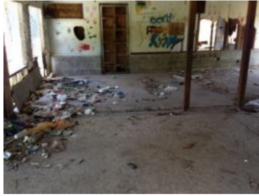
Photo 12 – Asbestos Debris in Old House
