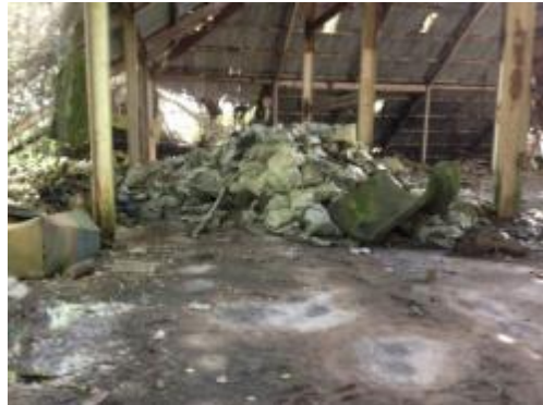
Photo 57- Abandoned Insulating Material
