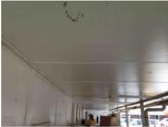
Photo 8 – Asbestos Hospital Parapet Ceiling
