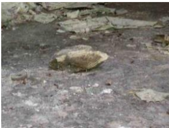
Photo 15 – Lump of Reported Asbestos
