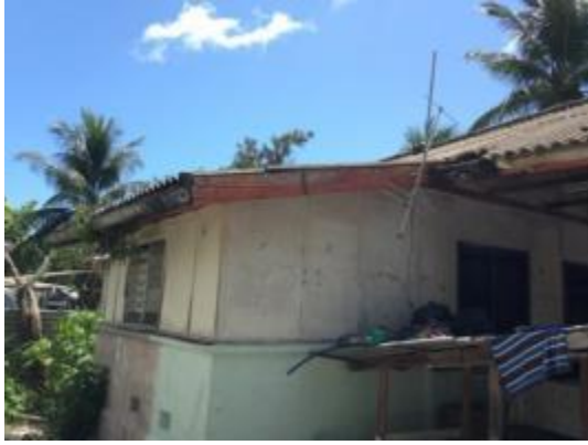
Photo 11 – Possible Asbestos Cladding
