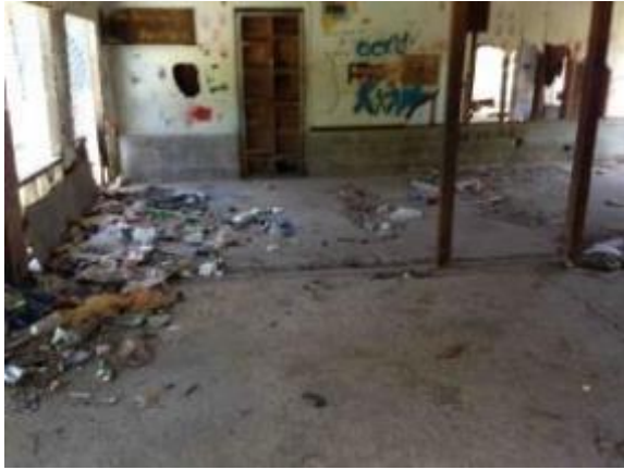
Photo 5 – Old House with Broken Asbestos
