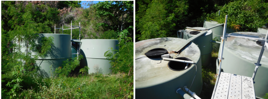
Figure 21. The older “Green” Sewage Treatment Plant at Nauru Primary School
