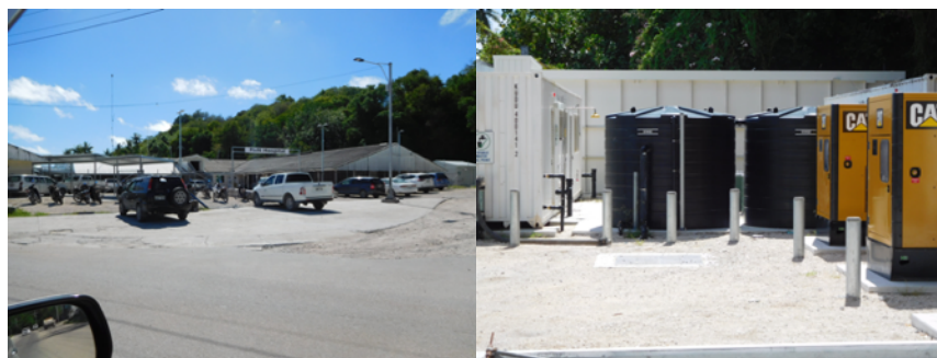
Figure 23. RON Hospital with Black Sewage Tanks (Right Hand Side)
