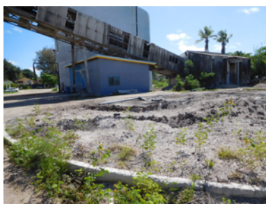
Figure 14. View showing remaining base of 'B10' and Upgraded Pump Station Building (Blue Building)
