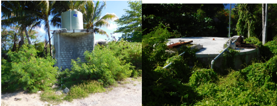
Figure 16. Water Storage Tanks for the Meneng Brackish Water Scheme
