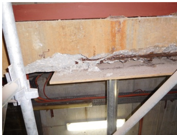
Figure 11. Concrete damage and exposed Steel Reinforcement on Upper Floor Slab
