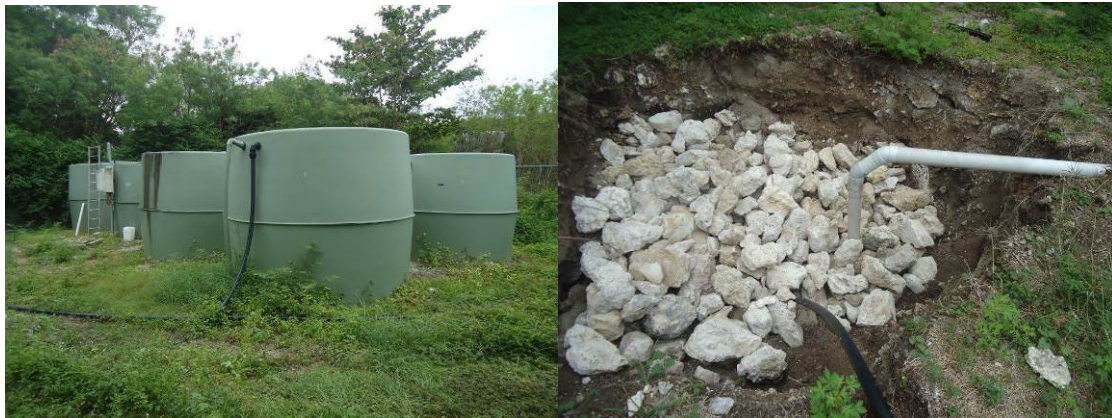
Figure 6. Sewage treatment Plant at Nauru Primary School with Effluent Dispersal Pit
