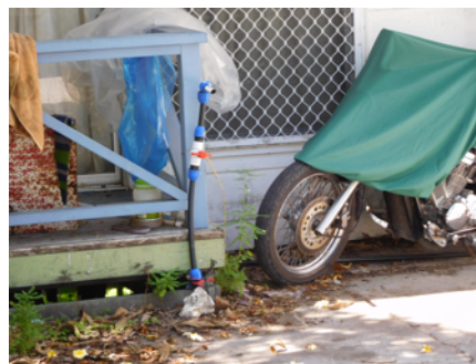
Figure 18. Typical Brackish Water Service Connection in Meneng
