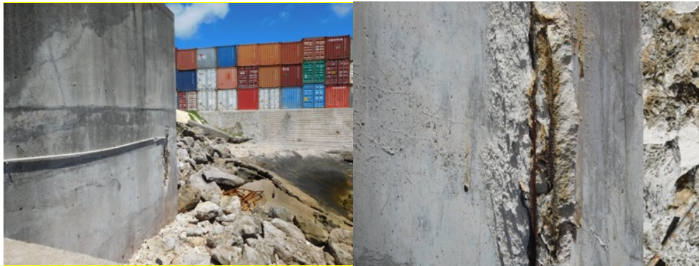
Figure 9. External Concrete Damage to Structure with Steel Reinforcement Now Exposed
