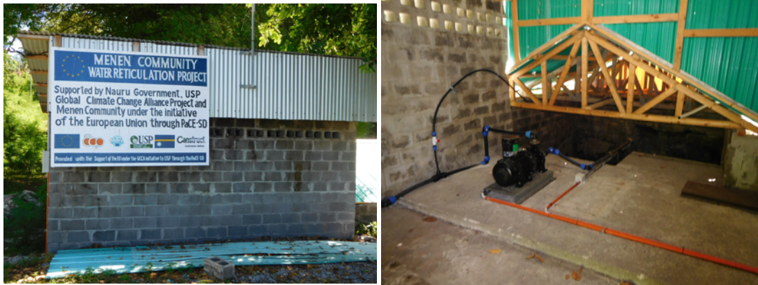
Figure 17. Pump Station for Brackish Water
