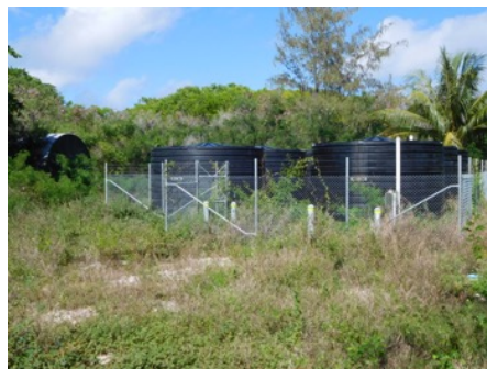
Figure 7. New Sewage Plant for New School Building at Nauru Primary School
