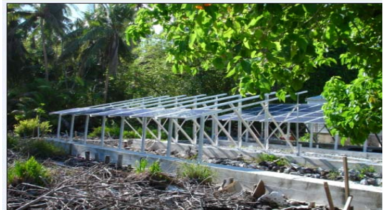
SOLAR ARRAY STRUCTURES
